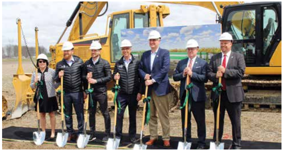
Breaking ground on Greenleaf Foods, SPC in Shelbyville (April 2019). It will be North America's largest plant-based protein manufacturing facility (H2O Design photo).
