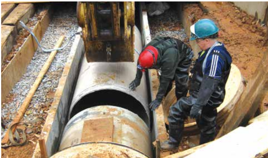
Safety is paramount at Midwest Mole. The trenchless technology company will expand its Greenfield headquarters this year and plans are underway to establish an office in Washington, D.C.
