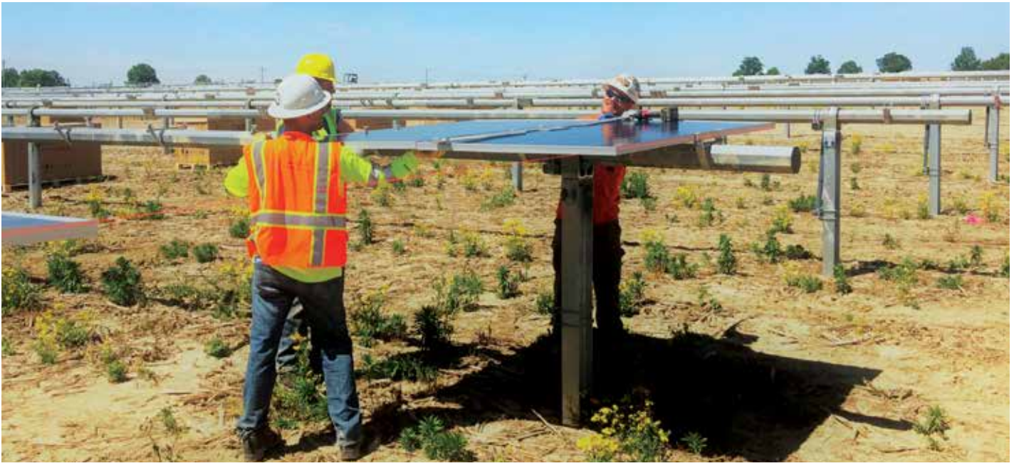
Hoosier Energy contractors install panels at a solar site on Interstate 74 near the Greensburg interchange. The 1MW array is one of three under construction and will be one of the 10 in the organization’s coverage area in southern and eastern Indiana ( Hoosier Energy photo ).
