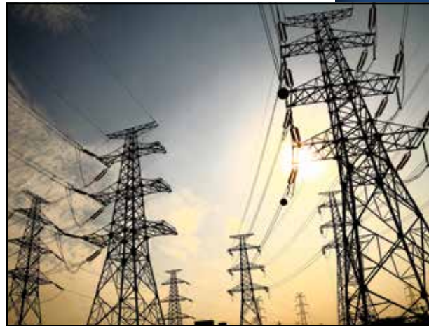
Substantial planning and permitting precedes development of any new transmission lines.
