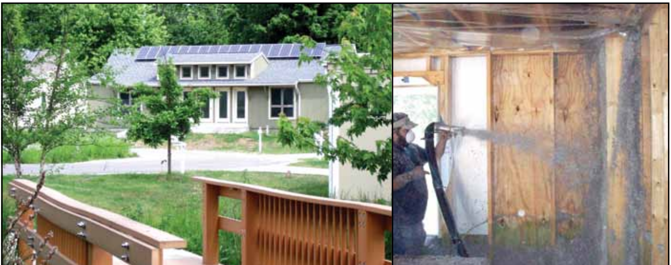
The city of Bloomington is offering housing that will save money on energy bills for low-income families. Recycled newspaper was used to insulate the walls of the 12-home subdivision.
