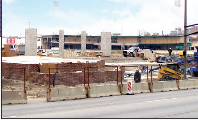
The under-construction Parkview Field baseball stadium ties into each element of the Harrison Square downtown revitalization project.
